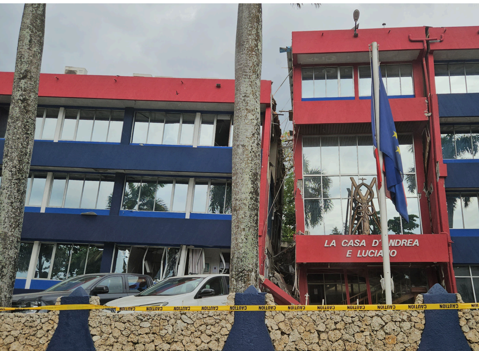
Picture 4: Building damaged
