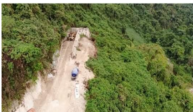
Brenwei Hydro Power Plant
